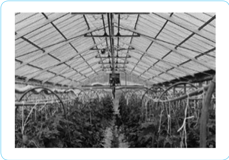
Figure 3-2 | Moving Spryer in a Greenhouse
