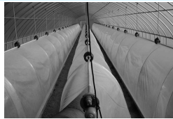
Automatic tunnel opener
